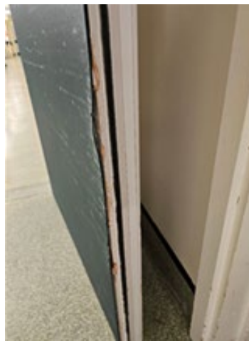
Example of damage to edge of fire door
