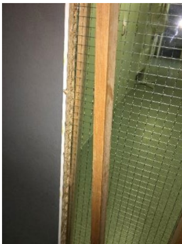
Example of damage around glazing
