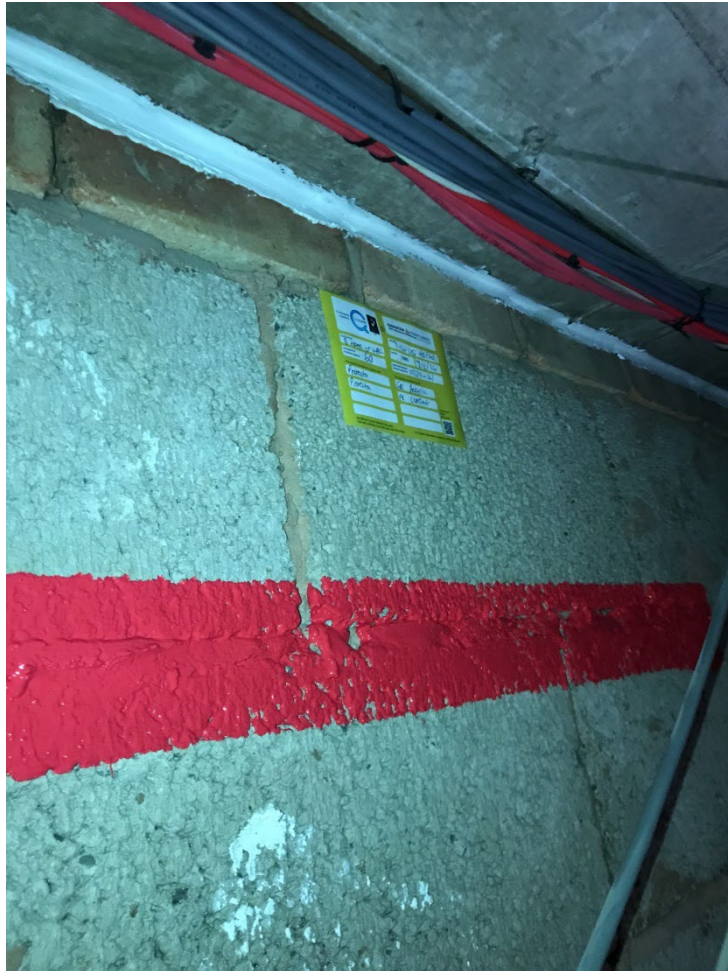
Painted Red Line on Fire Wall
